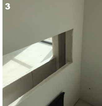
3 The fireplace wall is not secured against false draft in the sides.
